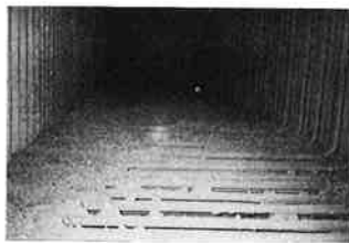
Secondary superheater (2SH)
